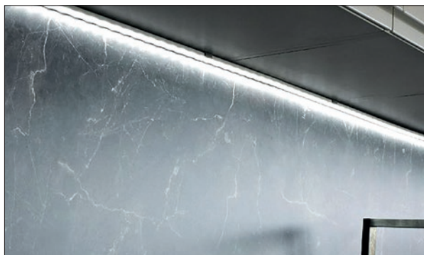
Wall Unit Strip Lights
